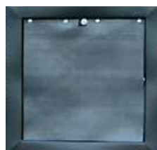
Return Air Vent
